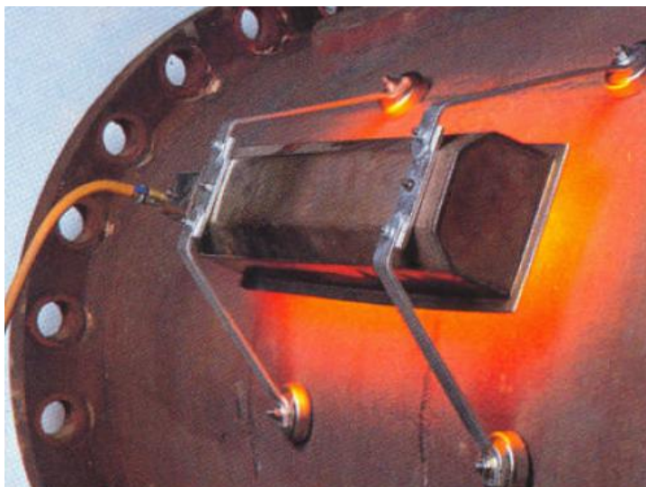
Infrared gas heater at vessel
